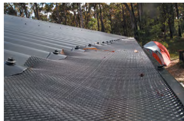
Metallic gutter guard. Source: Paul Whittington
