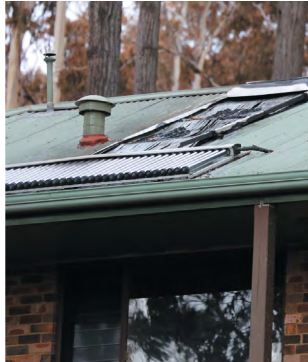
Example of roof perforation and combustible elements on roof. Source: CSIRO
