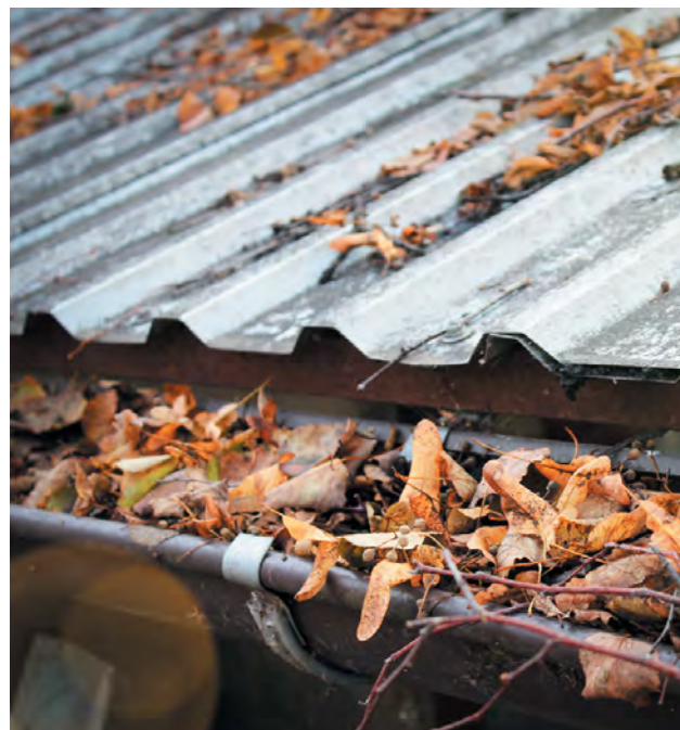
Debris accumulation in gutter.
