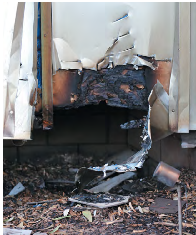
Damaged wall from burning vegetation. Source: CSIRO
