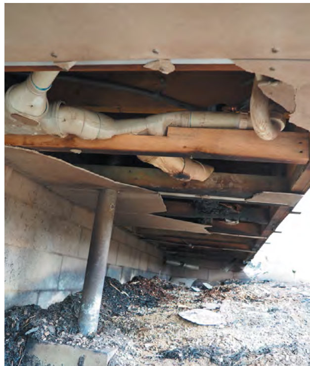
Underfloor damage caused by burning garden bed, suppressed by fire agency before it burnt into the house. Source: CSIRO
