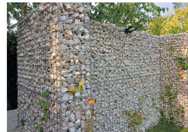
Non-combustible garden walls can protect against all modes of bushfire attack.
