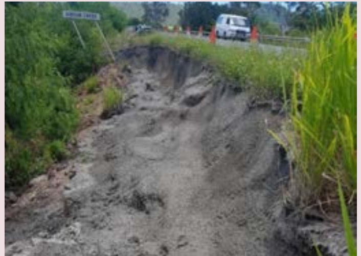
Bruce Highway (Mackay–Proserpine) – emergency works to stabilise the damaged slope with sprayed concrete (January 2023)
