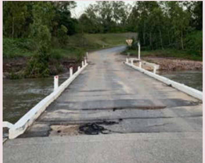
Laura River bridge – damage from Tropical Cyclone Tiffany (February 2022)
