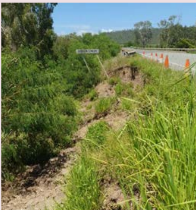
Bruce Highway (Mackay–Proserpine) – batter damage at Gibson Creek caused by Northern and Central Queensland Monsoon and Flooding event (January 2023)
