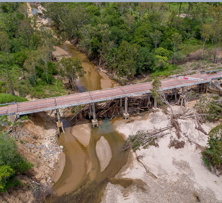
Image: damage from the Monsoon Trough event.
