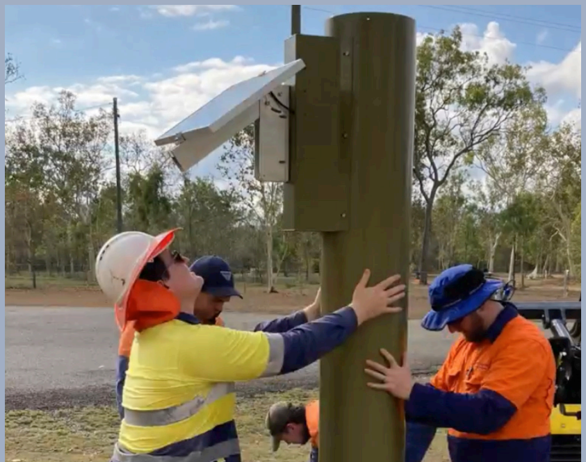
Image: Installation of valuable flood warning equipment under the Flood Warning Infrastructure Network (FWIN) Project kicked off in Townsville in mid October with the first rainfall gauge was installed in Oak Valley, south of Townsville.
