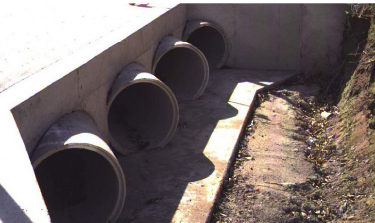
Images: (Top) Rifle Range Road Burdekin Shire Council damage. (Bottom) Rifle Range Road Burdekin Shire Council repaired.
