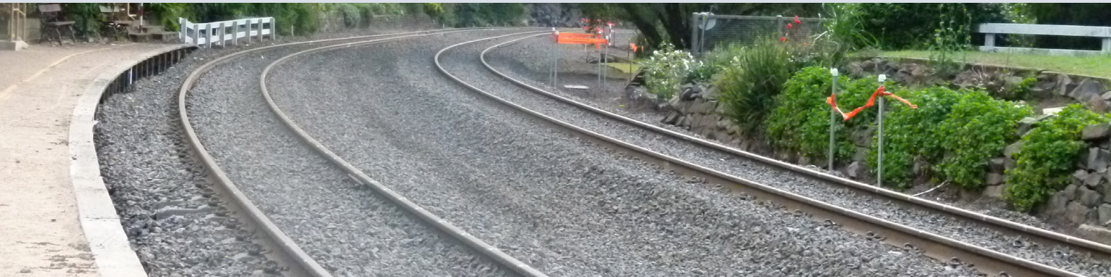
Images above: Queensland railway damage, during repairs and restored.
