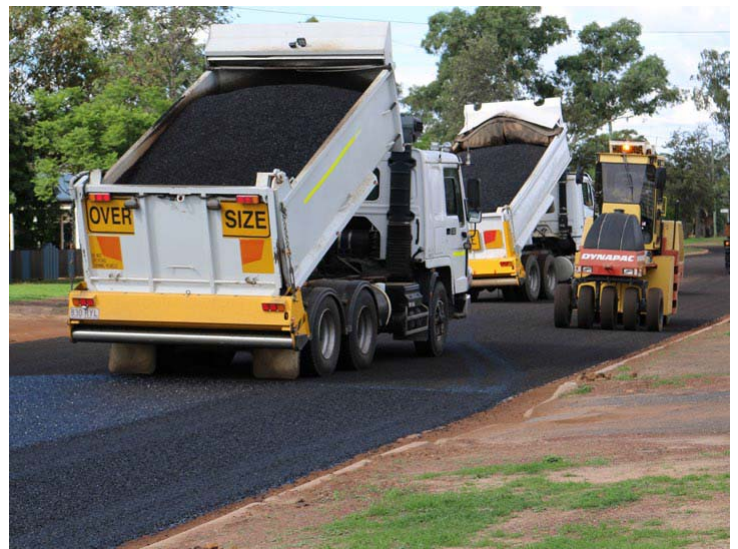
Alice Street in Dalby was a hive of activity as the final works were completed on Council's Operation Road Restore program
