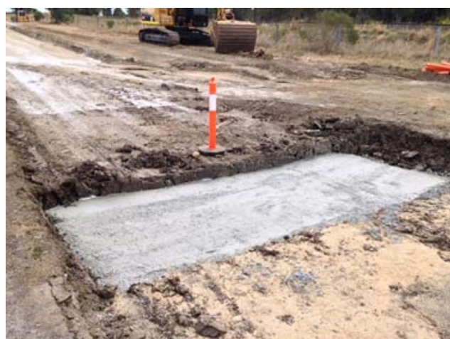
Right: Protective concrete slab over underground services on the Warrego Highway.
