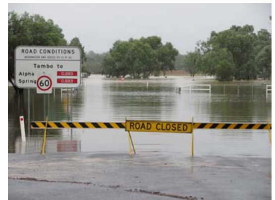
2010 disaster event damage to Esk–Hampton Road (top) and Barcoo River Bridge (bottom) - two reconstruction projects managed by the TNRP team
