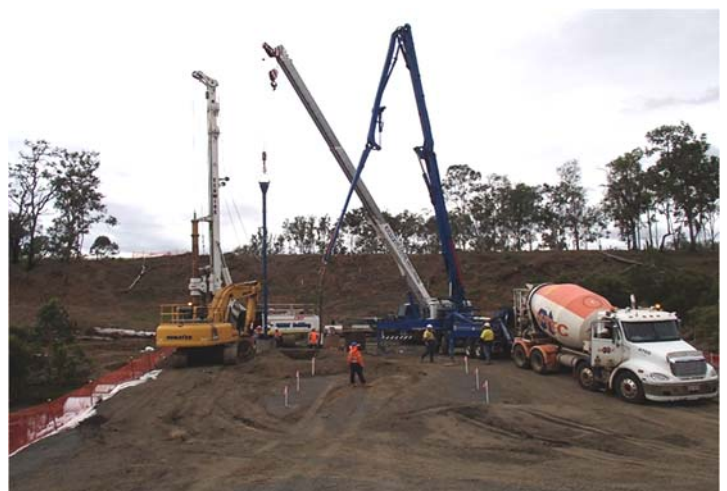
Opposite from top: Preparation for bridge approaches; Steel liner and reinforcement cage for piles; Drilling and pile installation from the temporary construction platform
