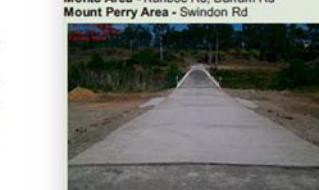
Bon Accord bridge approach, Gayndah. Council acknowledges the Natural Disaster Relief and Recovery Arrangements (NDRRA) funding is a joint Commonwealth and State Government program.
