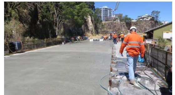
Above: girder mold in preparation for a concrete pour (top); concrete pour underway (centre); and the same girder after the pour has been completed (bottom)
