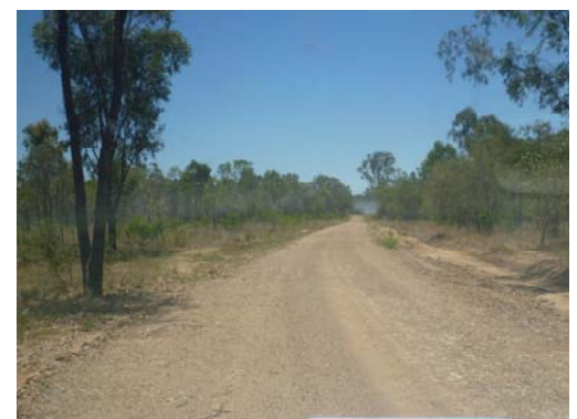
Above: damage (top) and completed works (bottom) to Five Mile Road, Woorabinda
