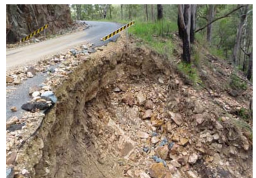
Above: landslide damage to Blackmans Gap Road, Gladstone Regional Council
