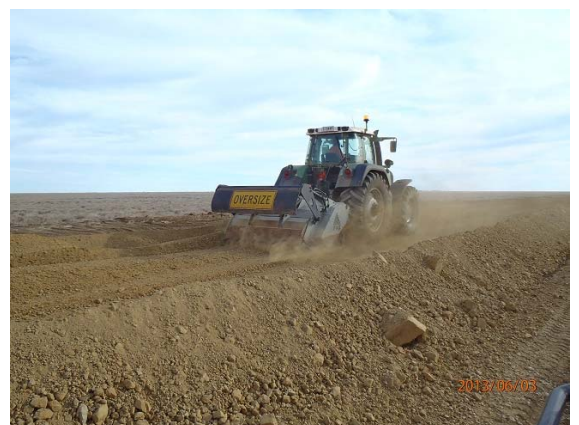
Above: damage to Ardrin Lane as a result of Cyclone Yasi related flood event (top); and during reconstruction works (bottom)
