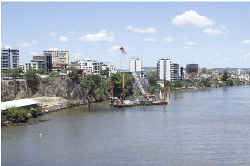
Above: the piling rig barge, with some of the piles in the background (Courtesy: Brisbane City Council)
