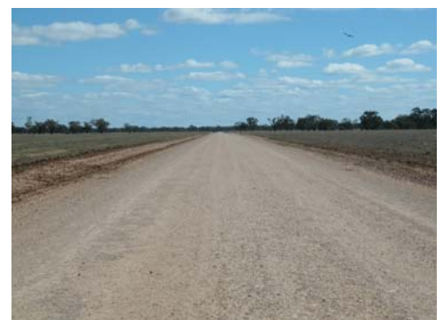
Right: Damage (top), works in progress (centre) and works following completion of a section of works (bottom) to Bulloo Downs Road
