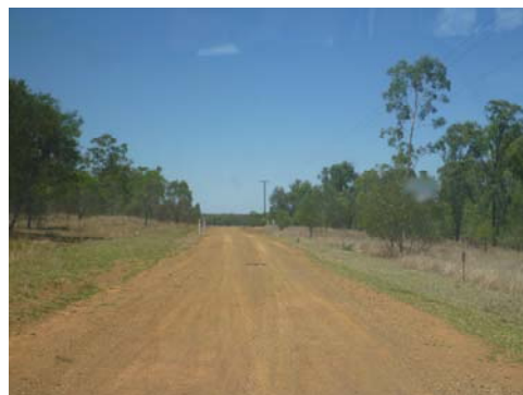
Left: examples of damage (left) and following reconstruction works (right) to Bore 3 Road, Woorabinda
