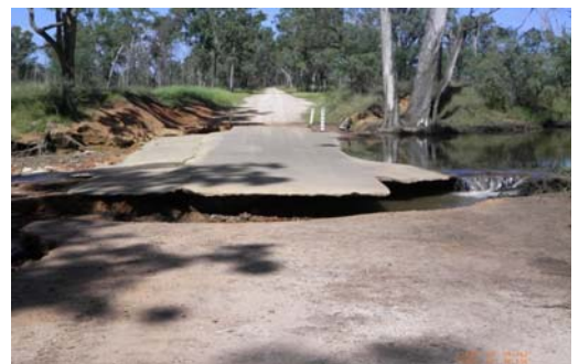
Above: undermining of concrete pavement slab and aprons - Conomarra Road, Central Highlands
