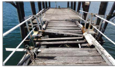
Above: Damage to Clump Point jetty.
