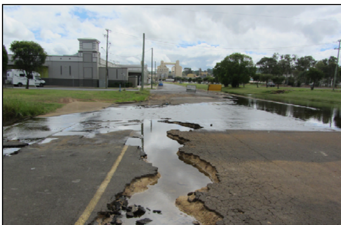
Above: Extensive pavement damage on Pound Street, Kingaroy (South Burnett Regional Council)
