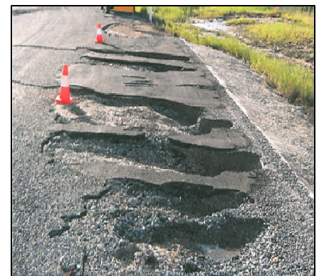
Above: Damage to the bitumen sealed floodway on Old Coach Road.
