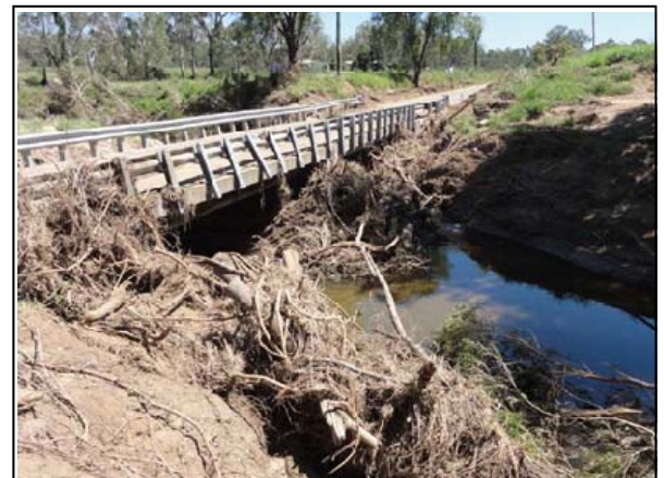
Above: Damage to Dairy Bridge (Lockyer Valley Regional Council)
