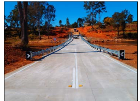
Above: Completed works at Mimosa Creek Crossing, including complementary funded crossing raising and installation of crash barriers
