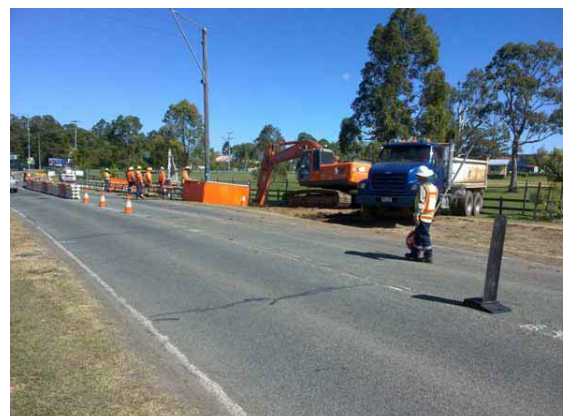
Right: works underway on Gregory Development Road (centre) and Mt Lindesay Highway, Beaudesert (bottom)
