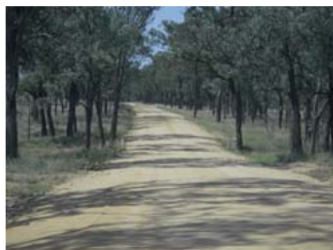
Left: damage (left) and following reconstruction works (right) to Defence Road, another of Banana Shire's roads damaged in the 2011 events
