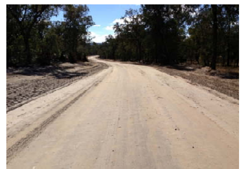
Right: Damage (top), works in progress (centre) and works following application of silty-sand/clay mix road base (bottom) to Mt Tabor Road
