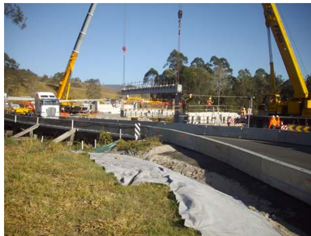
Left: Grigor Bridge ballast wall prior to pouring (left) and installing deck units in September 2013 (right).
