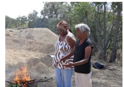
Top: Elder Doreen Jones explains the importance of the land for the Traditional Owners Centre: Traditional Owners, Doreen Jones and Carol Toby with SKM’s Matt Schlitz at the construction site Bottom: Doreen Jones and Carol Toby ask their ancestors to protect the contractors and staff for the project duration
