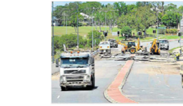
THE ONE MILE BRIDGE Damaged by the 2011 Flood. PHOTO: JARY UZNE
