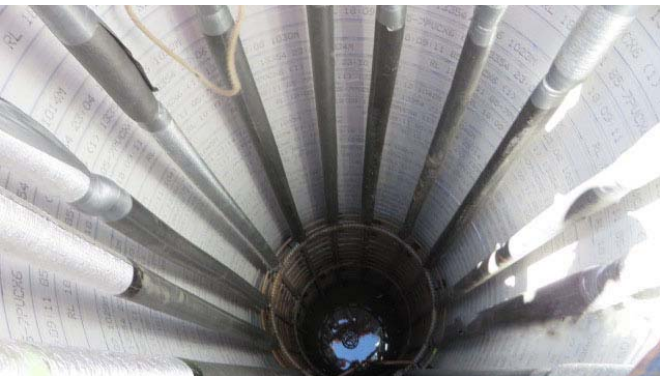
Above: Looking down inside one of piles before the concrete is poured; the steel bars are for reinforcement.
