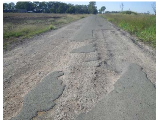
Above: damage to Jambin-Dakenba Road, one of nine roads approved for Betterment funding for Banana Shire Council.
