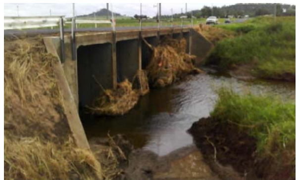
Damage to Kingsthorpe Haden Bridge as a result of ex-Tropical Cyclone Oswald in 2013
