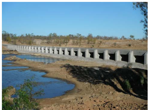
Completed betterment works to the causeways at Little Bynoe River (top), Bynoe River (centres) and Flinders River (bottom)
