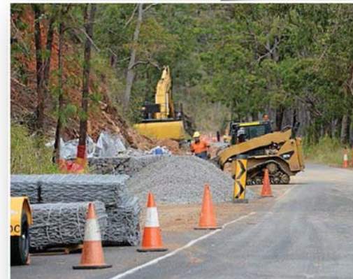
ROAD WORKS: It took 10 months to repair the damage caused by Cyclone Marcia to Pilbeam Drive. PHOTO: CHRIS ISON ROK10036CPILBEAM2
