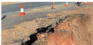
Cyclone Marcia causes major damage to Pilbeam Dr. PHOTO: CHRIS ISON ROK20035CPILBEAM4
