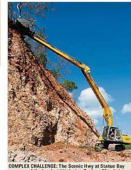
COMPLEX CHALLENGE: The Scenic Hwy at Statue Bay was one of the hardest hit during Cyclone Marcia in February. PHOTO: CHRIS ISON FOR QSLDRECONSTRUCTION.ORG
