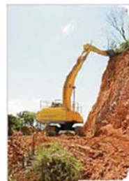
A large excavator works to clear loose rock and earth from the cliff adjacent to the Scenic Hwy near Statue Bay after Cyclone Marcia.
