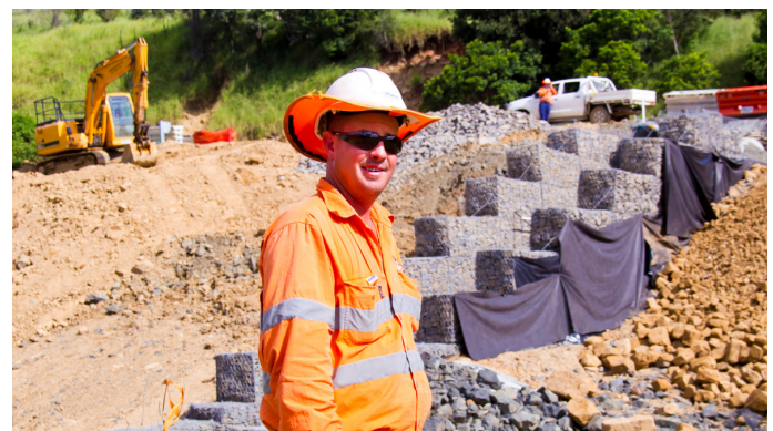
DTMR RoadTek contractors repair a section of the Warrego Highway between Marburg and Minden following the recent 2011 Brisbane floods
