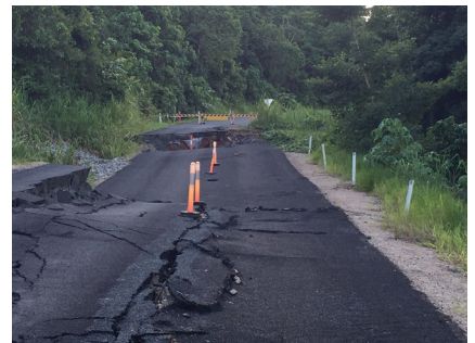
Tully Gorge Road impacted by the North Queensland flooding event in March 2018
